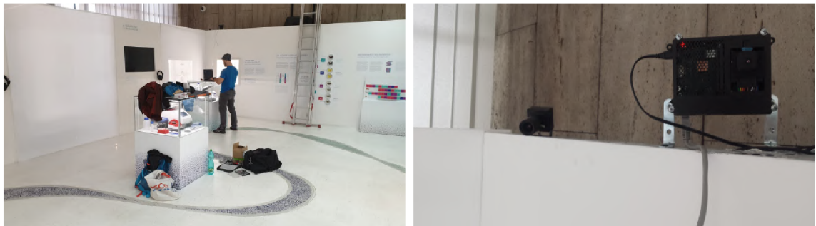
Figure 7.2: Illustration of the thermal unit installation process in the Czech National Museum in Prague.
