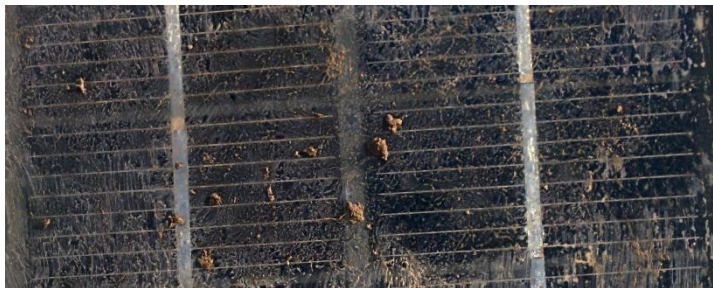
Figure 16. Contaminated PV panel (mud)
