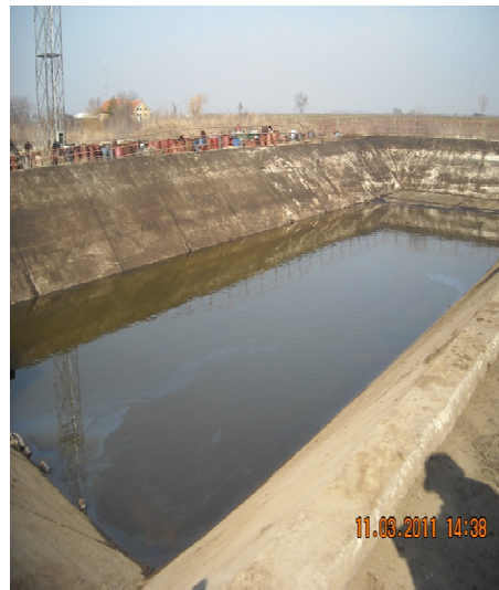
Photo 22. - Cleaned sedimentation tank after disposal of oil sludge in the Pancevo Oil Refinery (after) (source: www.nis.rs )
