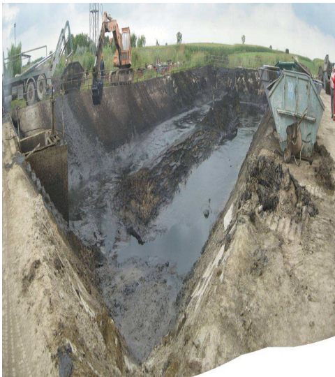
Photo 21. - Cleaned sedimentation tank after disposal of oil sludge in the Pancevo Oil Refinery (before) (source: www.nis.rs )
