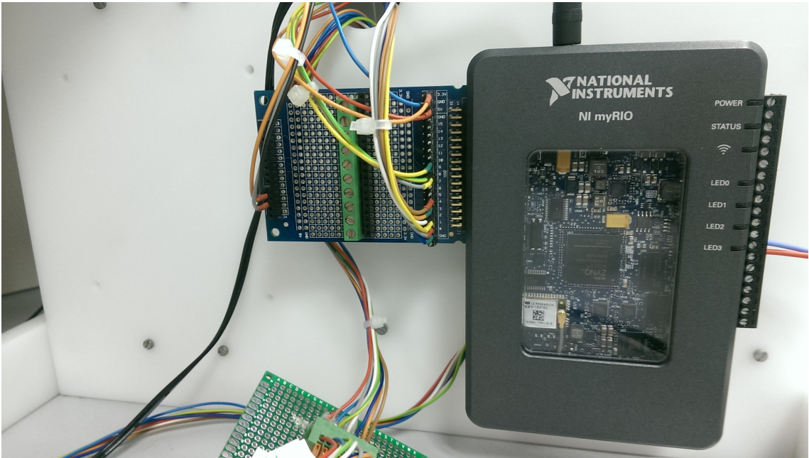
Figure 5.2: NI MyRIO with wired necessary connections.
