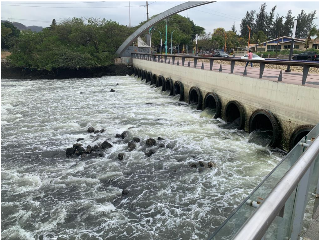
Figure 2.2: Photograph of the downstream side of Urdesa bridge and its flood control valves. Photo taken by Luis Dominguez.
