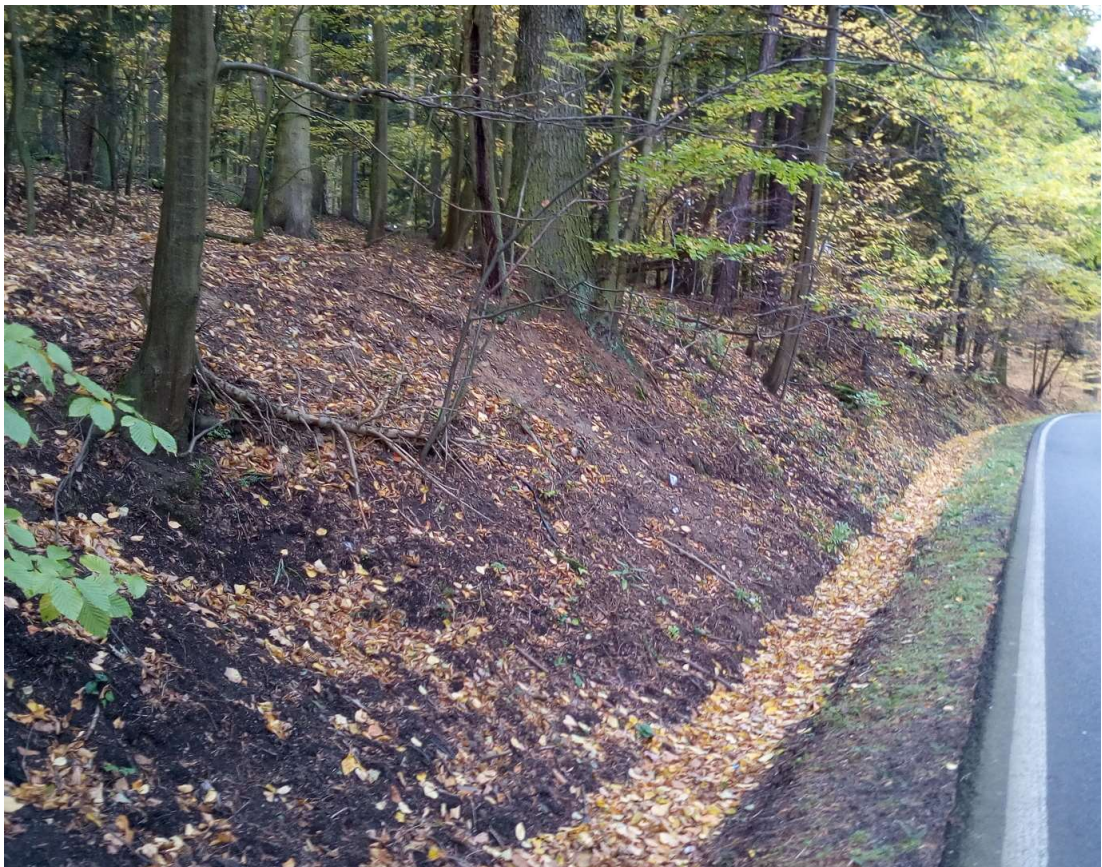
Figure 15. Eroded road side bank, location 1.
