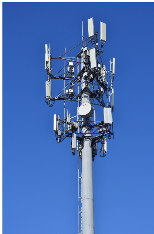
Figure 1.5: Top of a cellular tower
