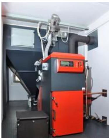
Obr. 11: Kotel Verner A251
