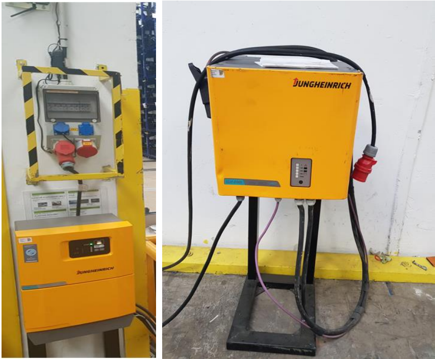
Figure 24: Chargers for Li-ion batteries (left – charger installed on the pillar, right – charger stand)
