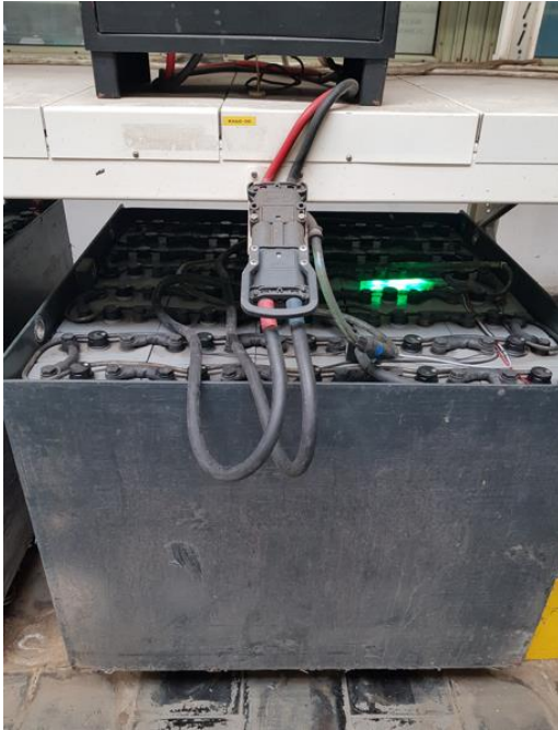
Figure 17: Lead-acid battery with a close look at the connector (demineralized water and electricity connector with a handle)
