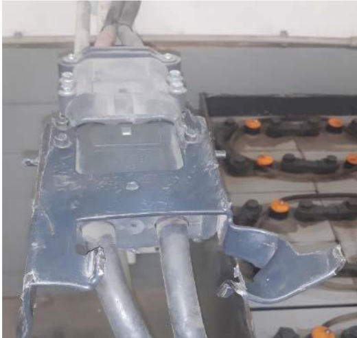
Figure 25: Damage to handle on a connector
