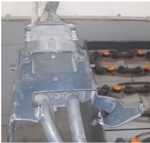
Figure 25: Damage to handle on a connector
