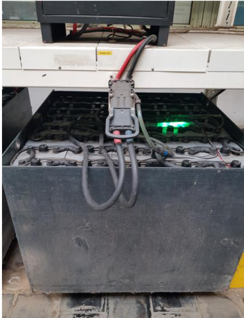
Figure 17: Lead-acid battery with a close look at the connector (demineralized water and electricity connector with a handle)
