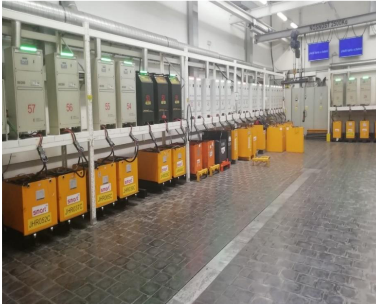
Figure 15: Charging station in Hall M2
