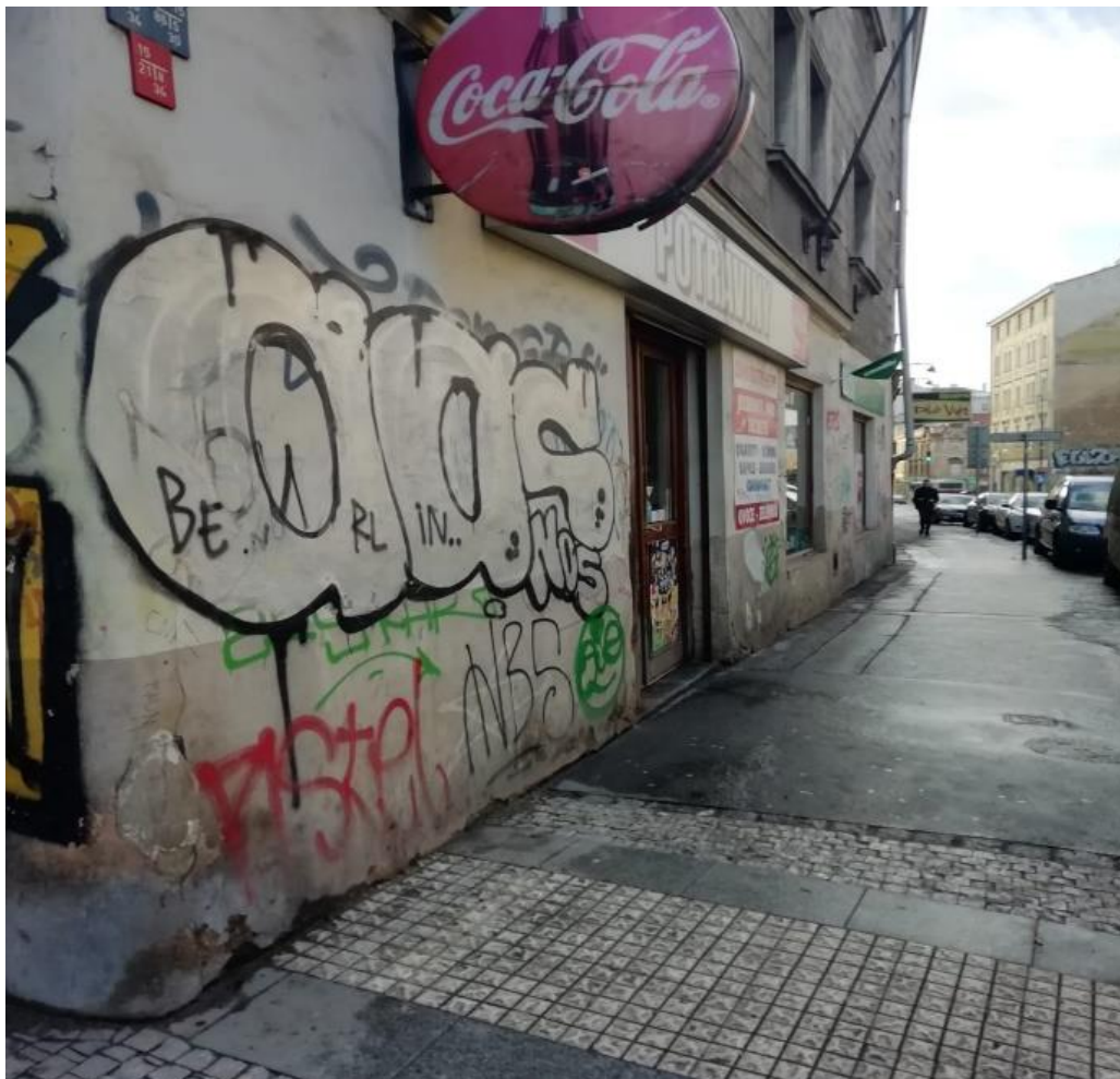
Figure 4.24: Showing a business outlet with heavily tagged wall
