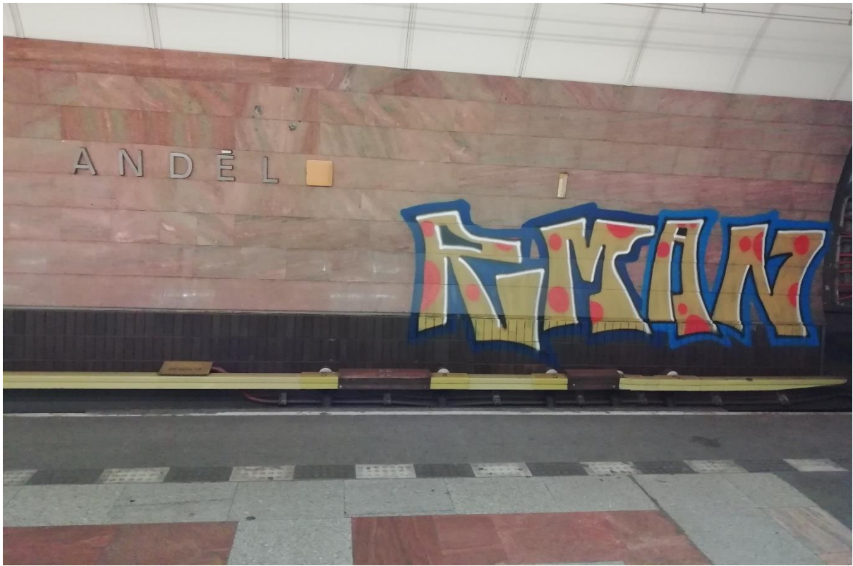
Figure 4.13: Showing graffiti on Andel metro station platform
