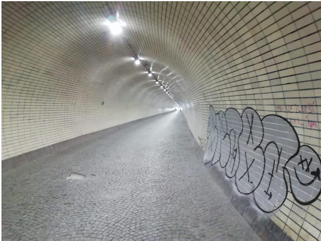
Figure 4.9: Showing graffiti on Zizkovsky tunnel's wall
