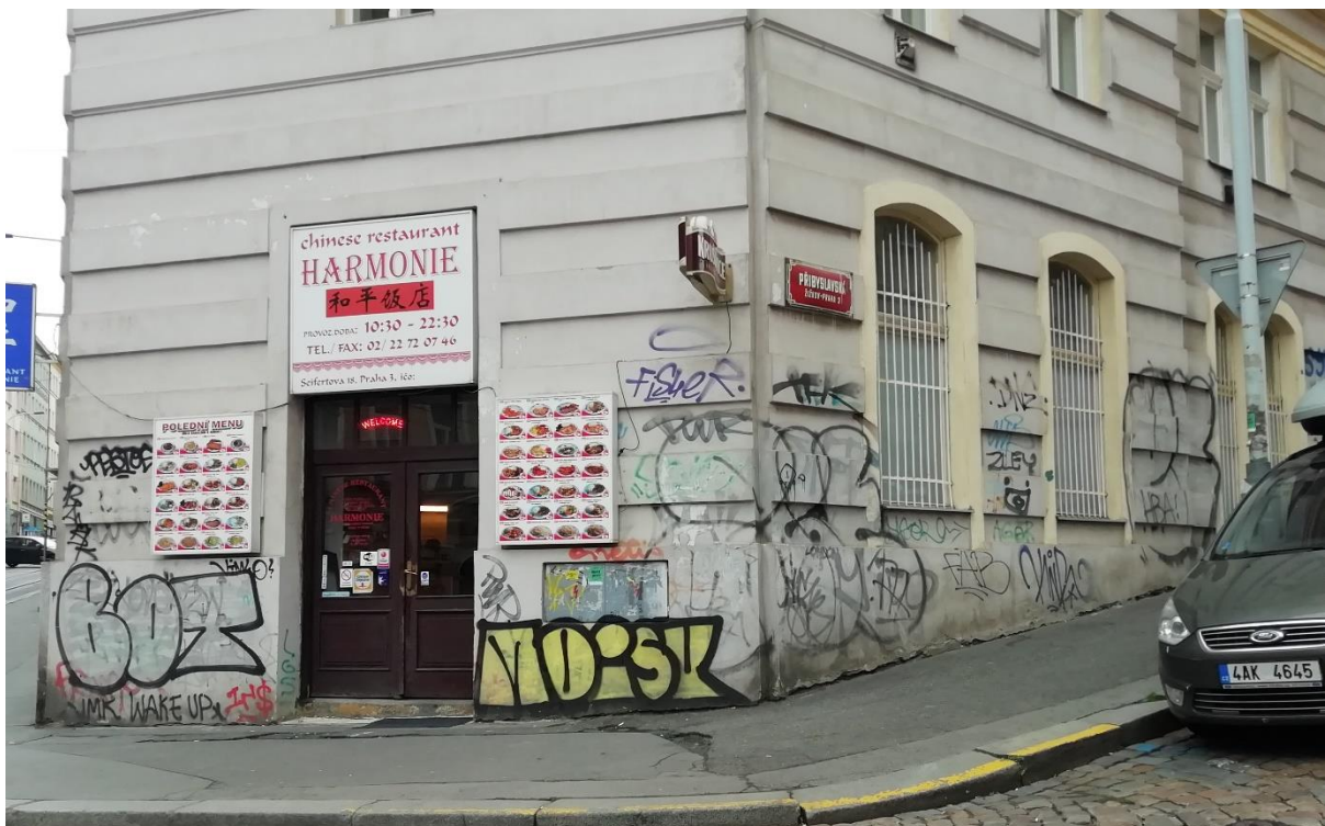
Figure 4.26: Showing a restaurant tagged with graffiti
