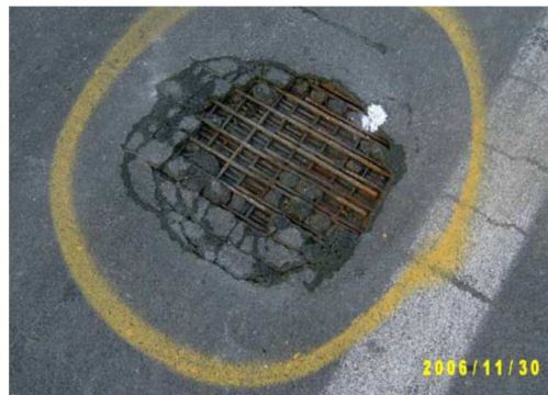
Figure 15: Dense reinforcement and badly compacted concrete [1]
