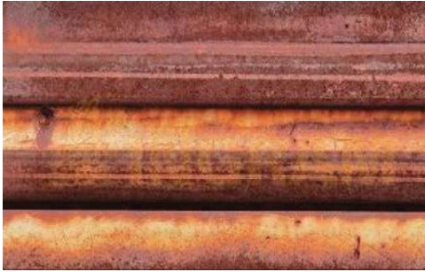
Fig. 6 High temperature corrosion. [7]
