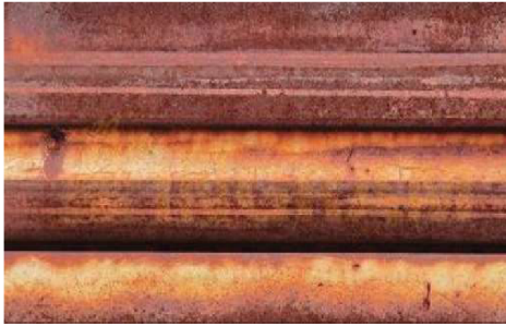
Fig. 6 High temperature corrosion. [7]
