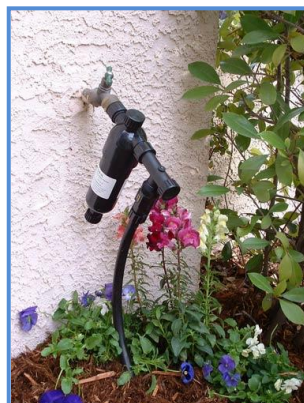
Figure 18.2 Drip irrigation system header
