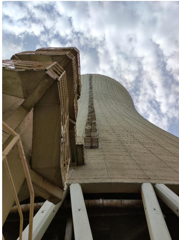
Figure 2. The cooling tower.
