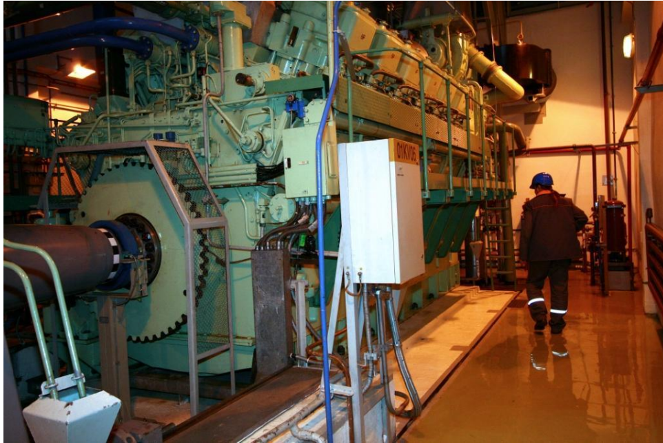
Figure 11. Diesel generator. Reprinted from ČEZ, a.s. (2012).
