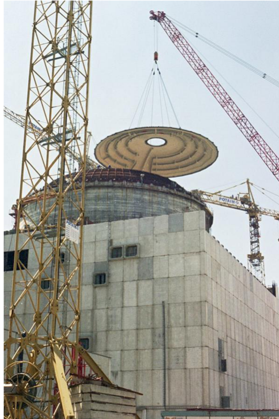
Figure 10. The spray system in the Temelín nuclear power plant.
