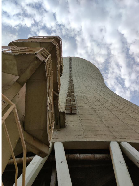
Figure 2. The cooling tower.
