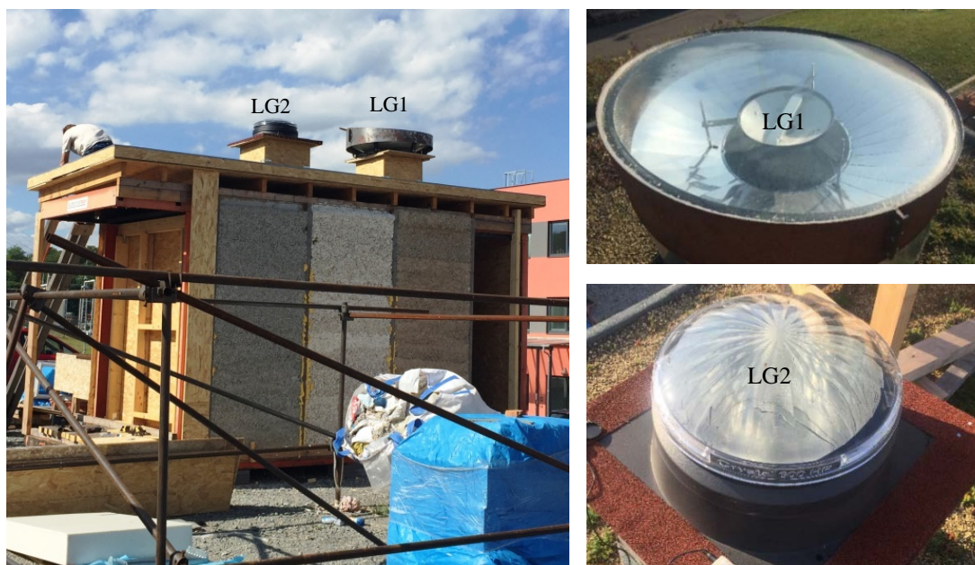
Fig. 3.27: Tested light guides LG1 and LG2 – the roof installation
