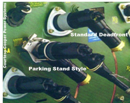
Fig. 3-24: Underground Circuit with Deadfront arrester. [2]
