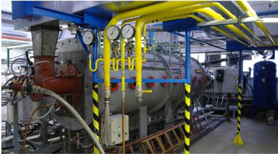
Fig. 20: Burner testing facility at Institute of Process Engineering [44]
