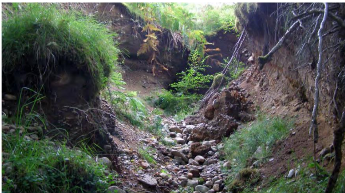
Figure 2. Excessive run-off has caused major erosion and gullying within this drain.
