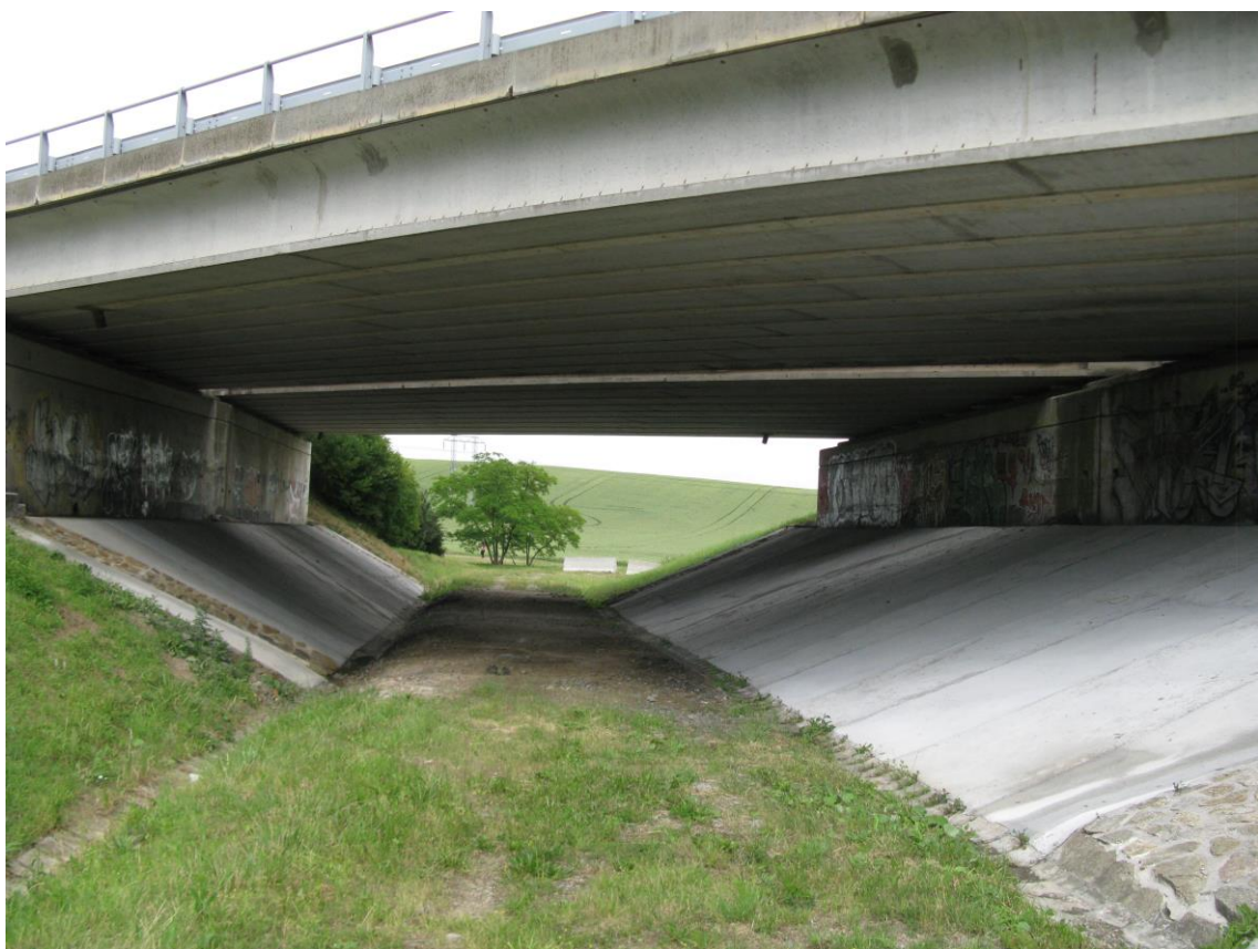
Fig. 22. Highway bridge over valley (Tučapy, D1 – 264 km), direction to south-eastwards from the D1 highway (27 th June 2015, photo of author)
