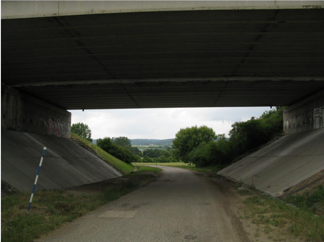
Fig. 21. Highway bridge over valley (Tučapy, D1 – 263 km), road direction towards Tučapy willage (27 th June 2015, photo of author)
