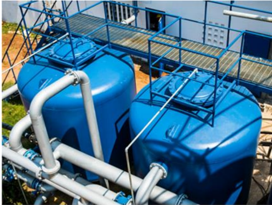
Figure 17. Water Treatment Plant at Akomnyada (source: Google image)
