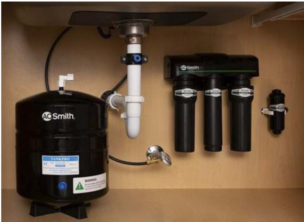
Figure 20. An Installed Reverse Osmosis System at Home (Google Image)
