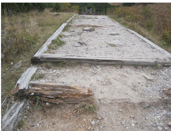
Figure 14 Erosion on trail to Labský důl (Photo: Author)
