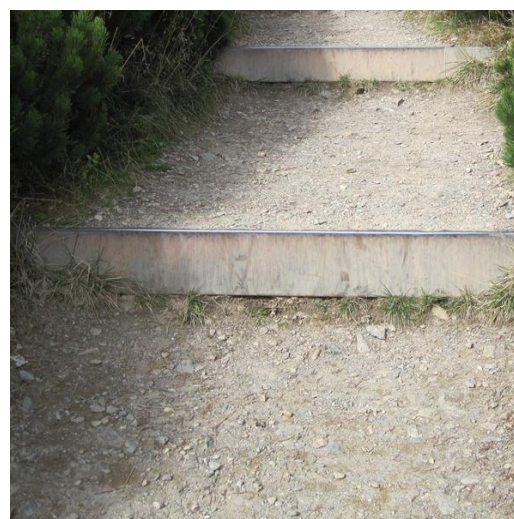
Figure 6 Trail to Snezka - eroded steps (Photo: Author)
