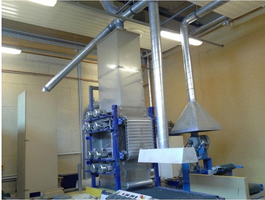
Figure 44 Installed inputs of a draught fan
