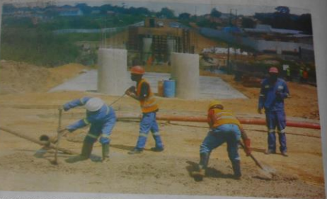
WORKS on the construction of the Mufuchani Bridge across the Kafue River.
