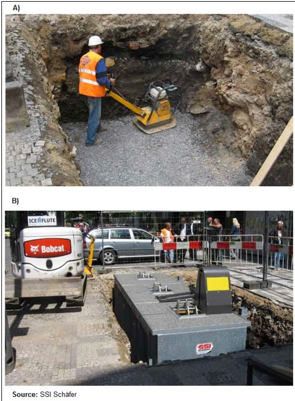
Picture 8 A) Preparation for the installation of underground containers; B) Placement of the underground containers
