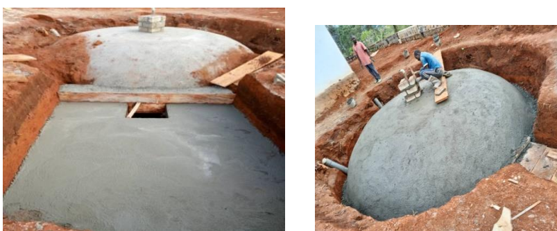
Figure 2: Construction of a 30 m 3 biogas in the mile 4 Nkwena slaughterhouse to be used mainly for cooking.
