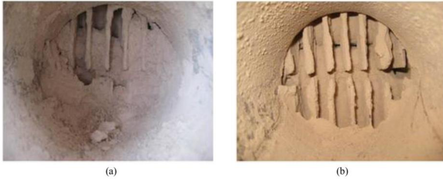
Figure 2: Actual pattern of ash deposition on H-type finned tube heat exchanger at different gas velocities after 18 hours at flue gas velocities (a) 4.5 m·s-1; (b) 6.25 m·s-1, for gas with high ash content. [2, p. 4683]
