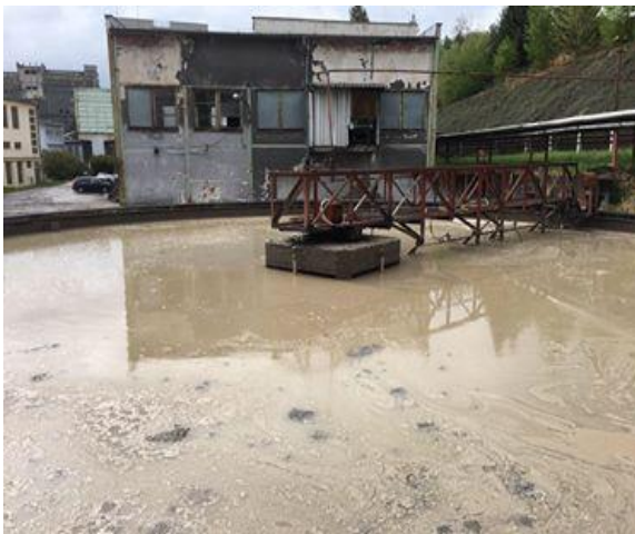
Figure 14: Sedimentation tank in JIP Větrní (Author 2020).
