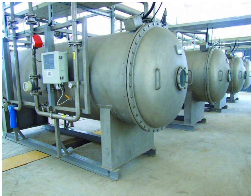
Figure 19: Industrial generator for wastewater treatment (Alibaba 2020).
