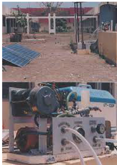
Figure 3.9: First mobile reverse osmosis unit established in Senegal in 1994, village camp of Palmarin, region of Mbour (preliminary studies carried out as part of a Senegalese-Japanese project, University of Dakar, EPT, 1993).
