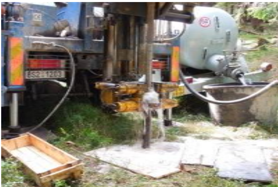
Appendix v: Drill core photographs on devices for mechanical work II (photo: AUTHOR)
