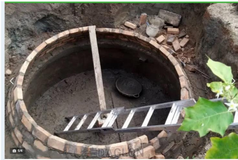
Figure 9: A biogas digester under construction in Ghana (source: Taken online from DAGLON-TECH, Ghana).
