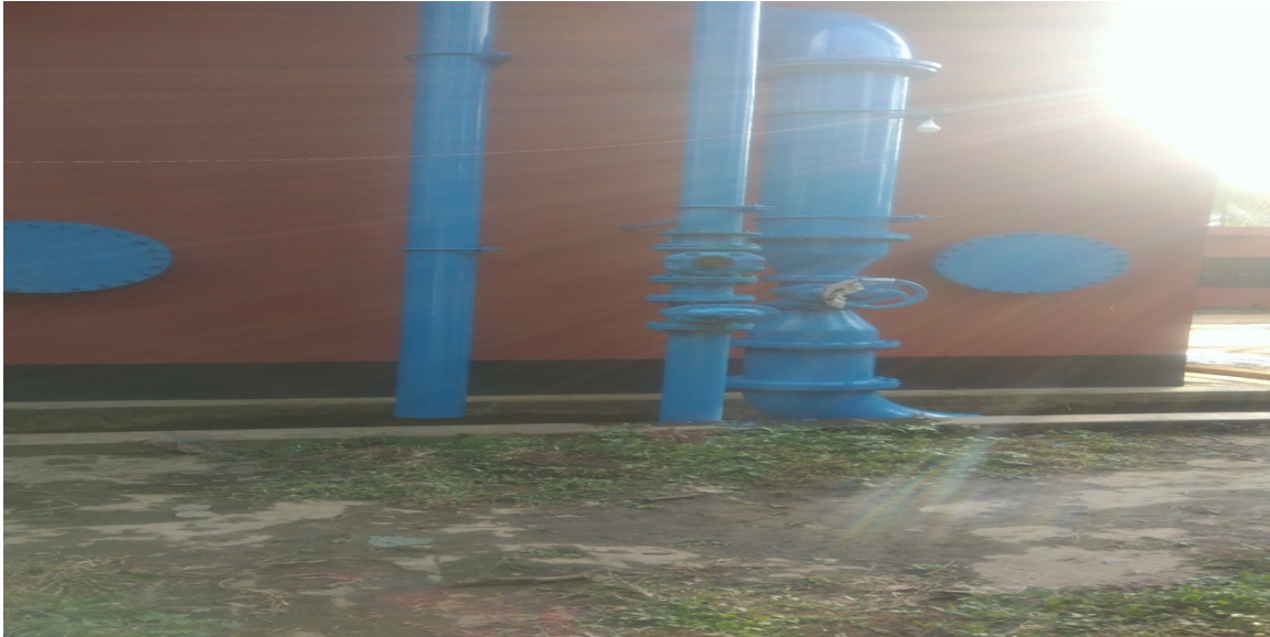
Figure 15: The residues from the sand filter tank (deferrization units) are drain out from the WPP
