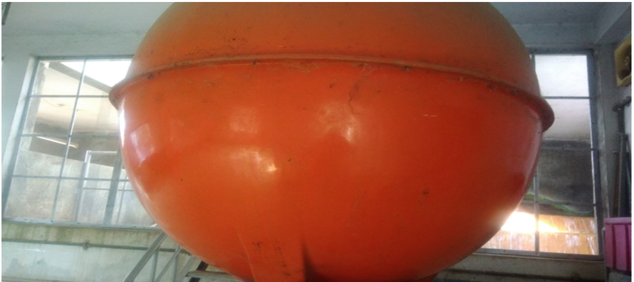
Figure 14: Sand filter tank
