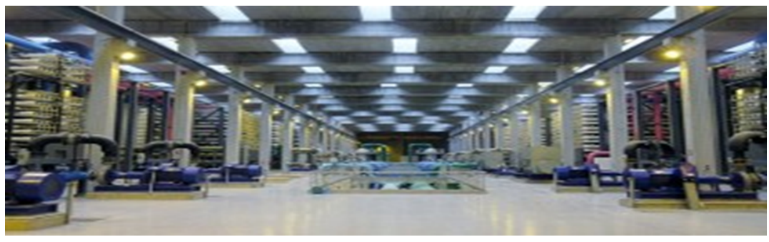
Figure23: Reverse Osmosis Technology
