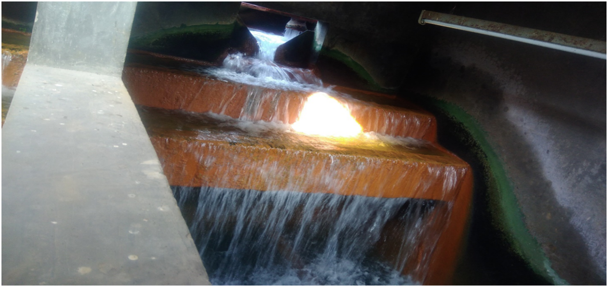
Figure 13: Water deferrization unit of water purification plant (WPP)
