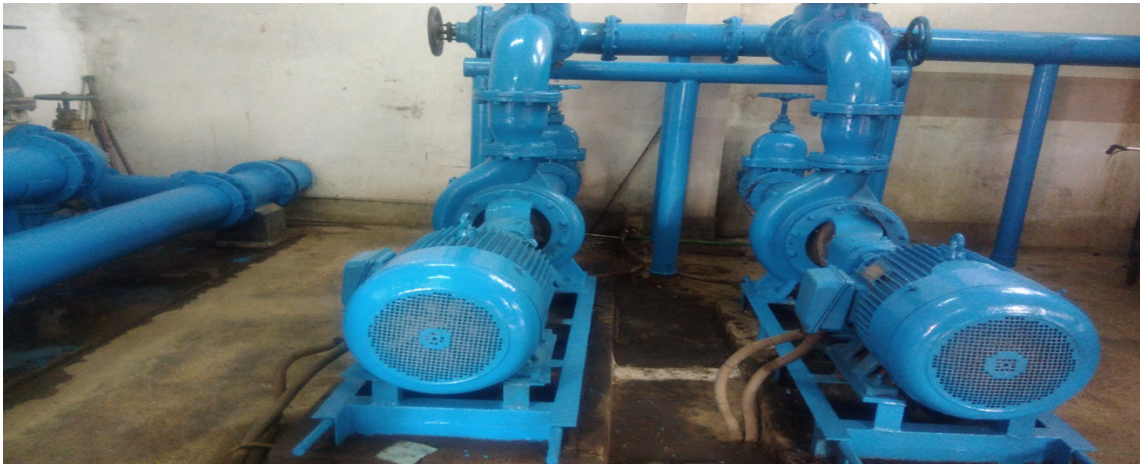
Figure 11: The untreated water from the underground wells is supply to reservoir by the set of centrifugal pumps.
