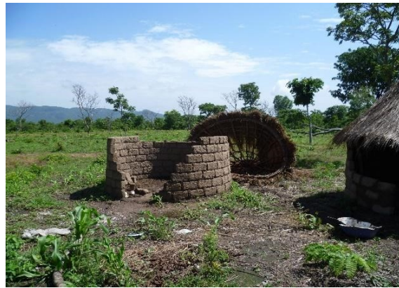
Figure 3 House damaged by elephant.
