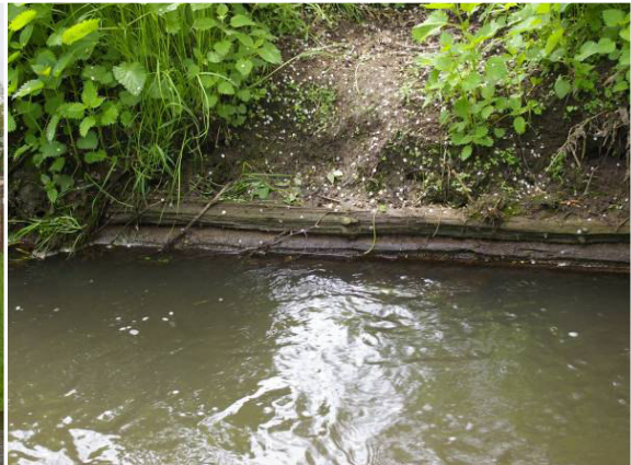
Figure 26: Lattice fence enforces the banks in between village Neuměřice and Kamenný most
