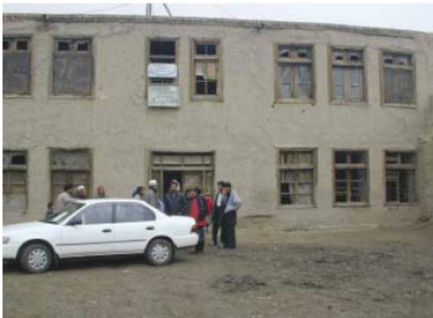
A dilapidated school in Kabul; some 80% of Afghanistan's school buildings are damaged or destroyed.
