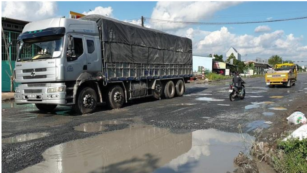
Image 2. Cai Lay bypass road (Tien Giang province) is seriously degraded
