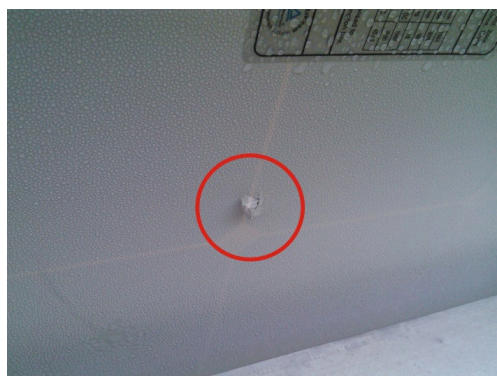
Figure 13. Mechanical damage to PV panel caused by chucked stone [25].
