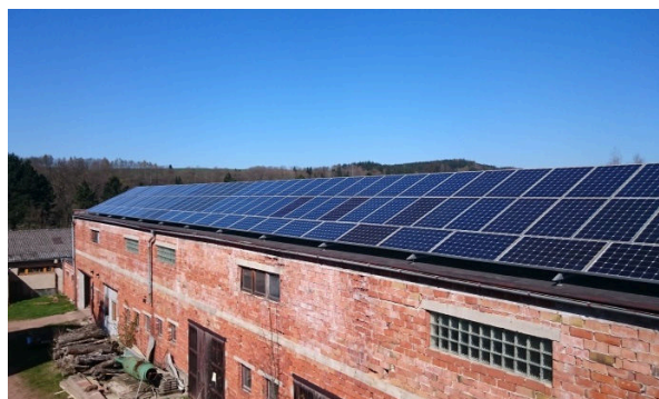
Figure 15. Selected part of the 100 kWp PV plant [27].
