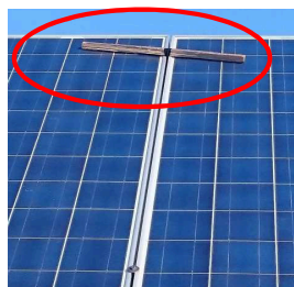
Fig. 4 Improper panel mounting
