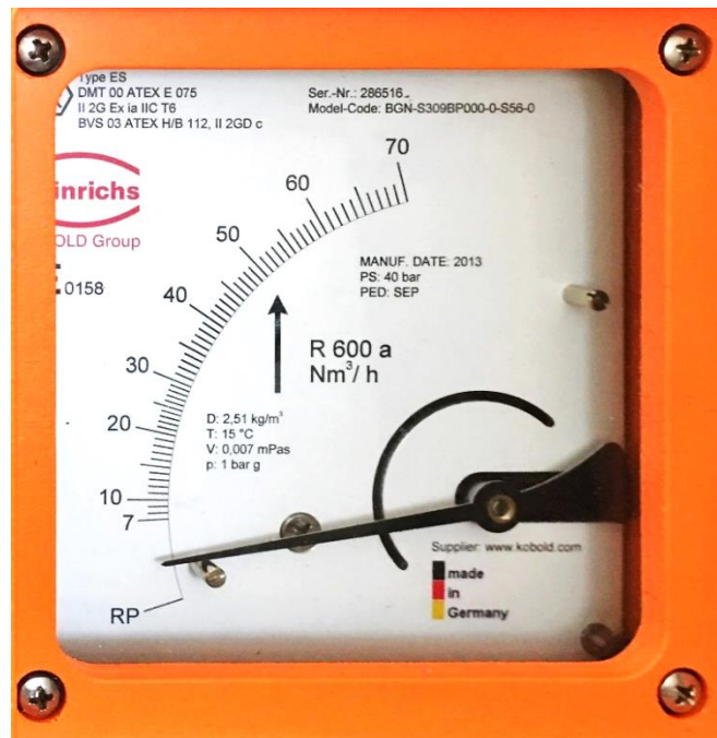
Figure 4.11 Analogue display of the variable area flowmeter at the ejector outlet.
