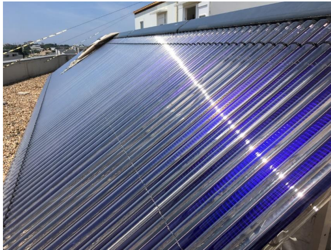
Figure 4.3 The four evacuated tube type solar collectors installed in series.
