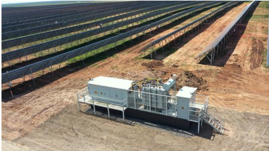
Figure 7 Nura Solar Power Plant [48]
