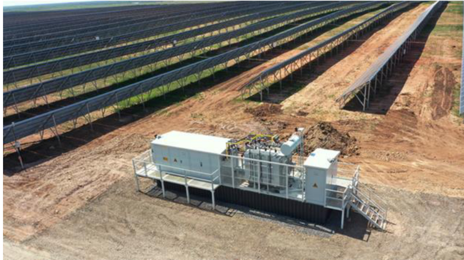
Figure 7 Nura Solar Power Plant [48]
