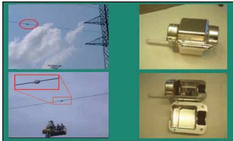
Figure 2-7 Typical installation on 220 kV line in Belgium (2005) [1]
