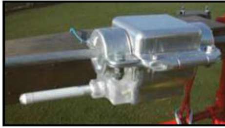
Figure 2-2 Typical installation on live line in France at 90kV on HT ACSS conductor [1]
