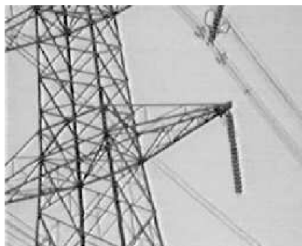
Figure 3-10 Damage due to galloping on a string of suspension insulators [2]
