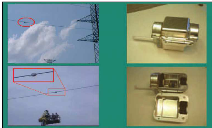
Figure 2-7 Typical installation on 220 kV line in Belgium (2005) [1]
