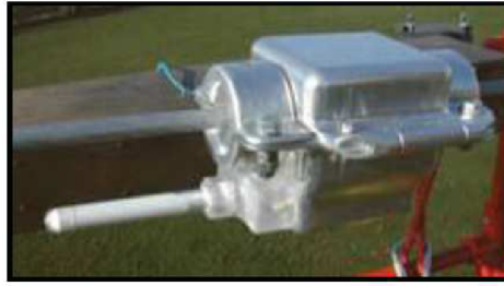
Figure 2-2 Typical installation on live line in France at 90kV on HT ACSS conductor [1]
