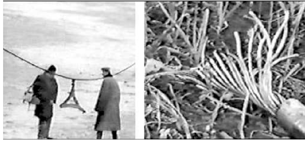
Figure 3-11 Damage due to galloping on a triple bundle conductor in China [2]
