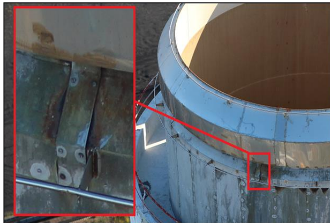
Figure 16. Cracks in a chimney. Reprinted from https://forcetechnology.com/en/articles/inspection-using-drone-technology
