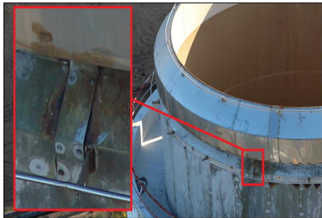
Figure 16. Cracks in a chimney. Reprinted from https://forcetechnology.com/en/articles/inspection-using-drone-technology
