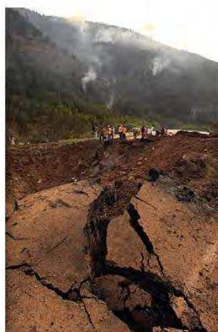
Crater and damaged roadway
