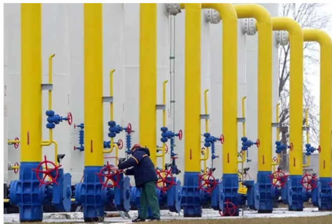
Figure 8: A Ukrainian operator at the main pipeline in the village of Boyarka, near Kyiv.
