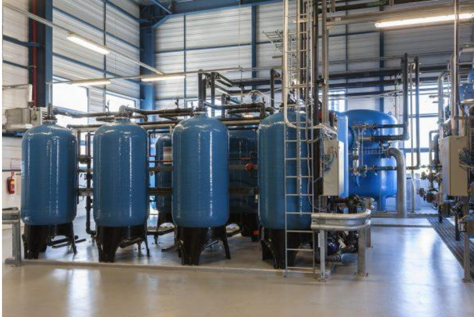
Figure 10 Ion Exchange Plant
