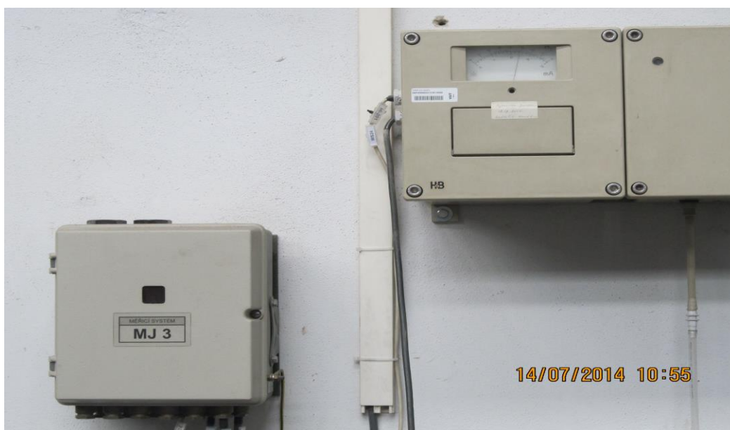
Figure 18 :Connecting the measuring units MJ3 (used only for measurement hydrogen content in the produced gas -online measurement)
