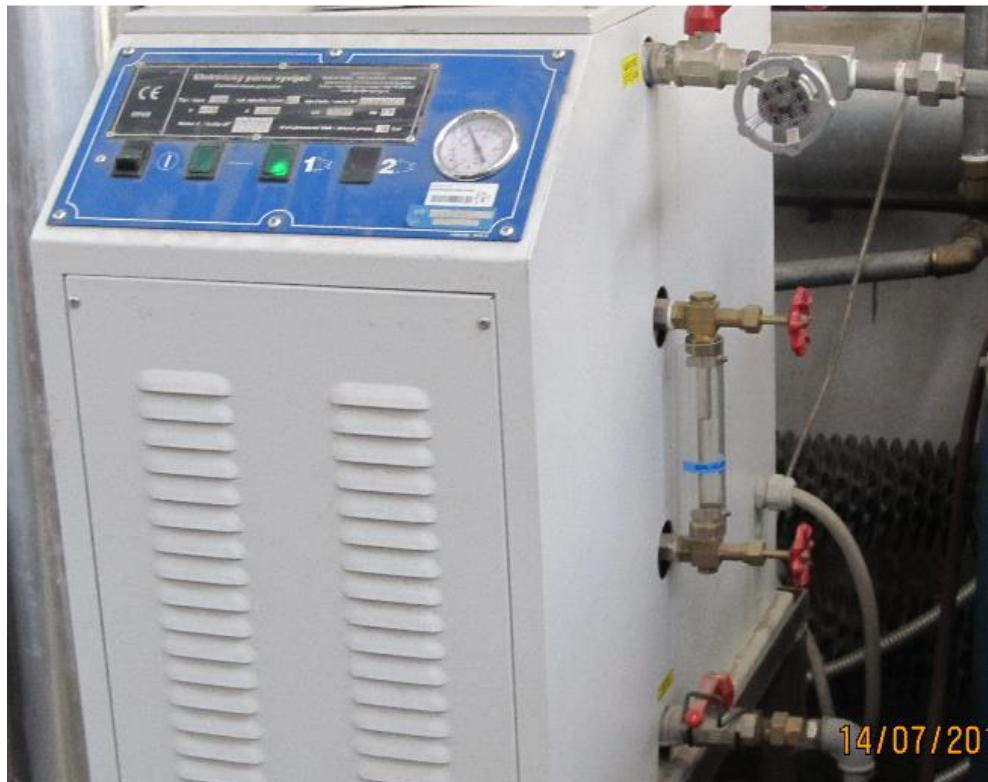
Figure 15: electrical steam generator
