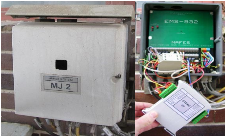
Figure 17: Measuring units MJ2 in laboratory (outdoor installation)
