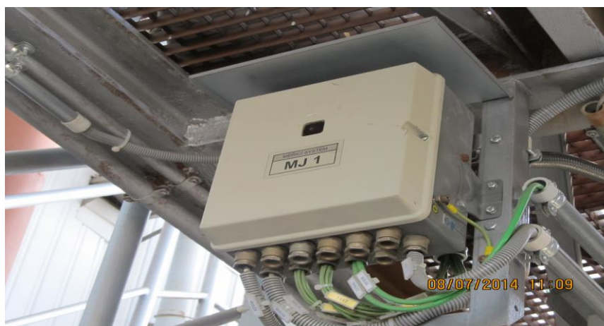
Figure 16: Measuring units MJ1 in laboratory (outdoor installation)
